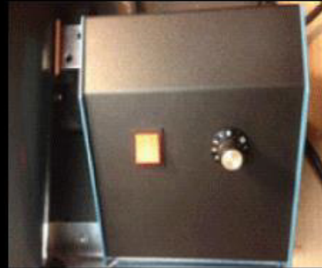
MOTOR CONTROL BOX
